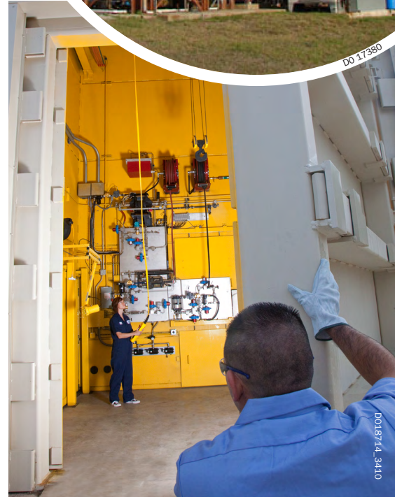
All high-pressure tests are conducted within large containment chambers to allow for safe operation.
